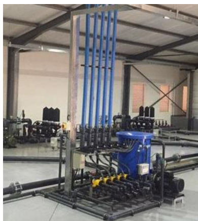
Figure 8-13. Picture of automatic fertigation equipment with mixing tank and vertical pipes ( https://pbs.twimg.com/media/DFIXyzUUQAEiEL.jpg )
