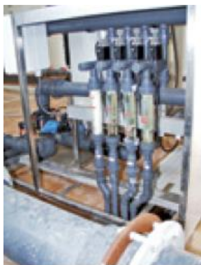
Figure 8-10. Installation of Venturi injectors inserted in a linear collector (Source: J. Antonio Marhuenda)
