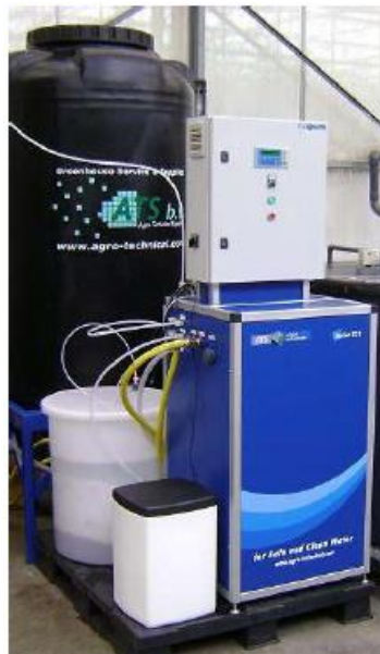
Figure 6-7. Installation for ECA water (Hortiplan)
