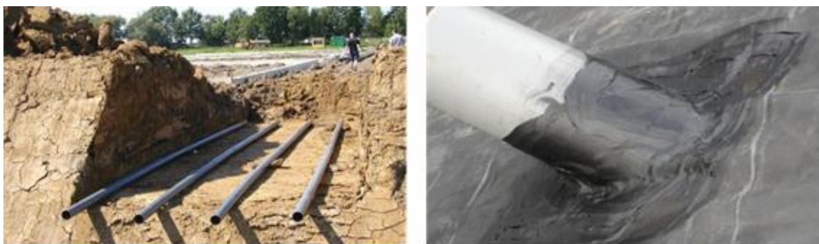
Figure 2-6. Installation of a waterproof pipeline through one of the dikes (Source: PSKW)
