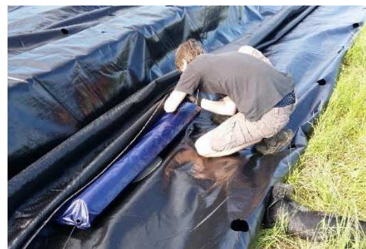
Figure 2-32. Ballast is attached to the vertical slabs, attached all around the floating horizontal foil (Source: PSKW)
