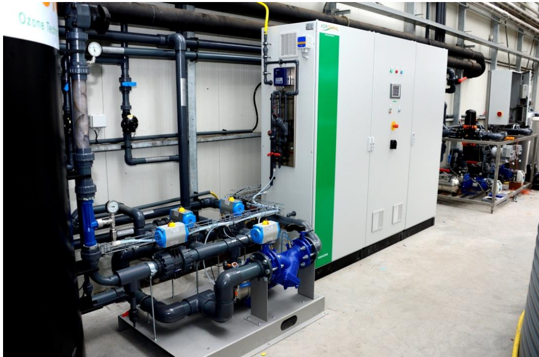
Figure 6-5. Ozone installation for horticultural water treatment ( https://www.glastuinbouwwaterproof.nl/ )
