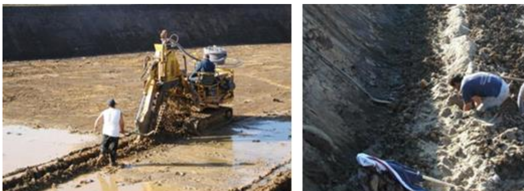
Figure 2-2. Left: Installation of the drainage system underneath the bottom of the water reservoir. Right: Drain tubes of coco fibre are placed in the gutters. The gutters are filled with sand to assure a good drainage of the groundwater (Source: PSKW)
