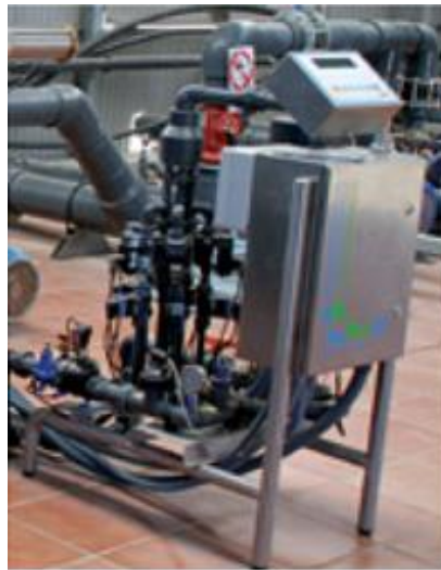
Figure 8-11. Installation of Venturi injectors in a circular configuration (Source: J. Antonio Marhuenda)
