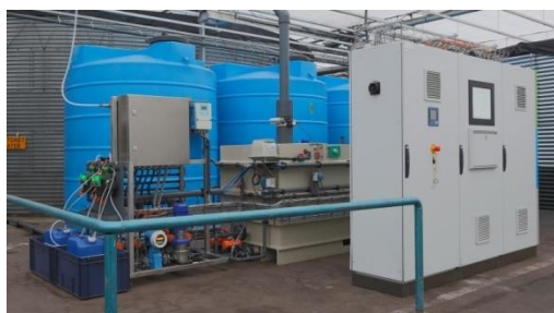
Figure 3-10. An example of a pilot installation for electrophysical precipitation in a horticultural greenhouse
