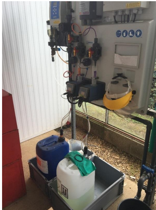
Figure 6-2. Sodium hypochlorite injection system using an electric pump and reservoir water at a UK ornamental nursery
