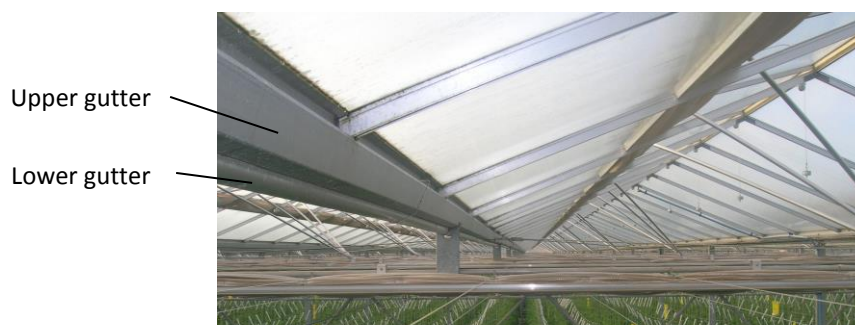
Figure 2-40. Picture of Venlo-type greenhouse with a double gutter for condensed water collection (Source: Santiago Bonachela)
