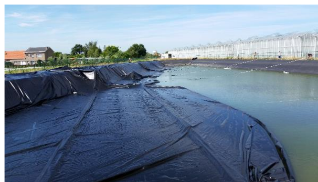
Figure 2-33. Manpower is needed to put the foil in its final position, so installation takes some hours (Source: PSKW)
