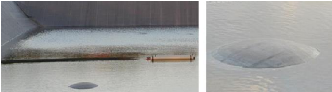
Figure 2-3. Bubbles indicate the presence of water or air underneath the foil. In case bigger bubbles are formed, this can lead to the rupture of the foil. Water underneath the foil also can harm the dikes (Source: PSKW)
