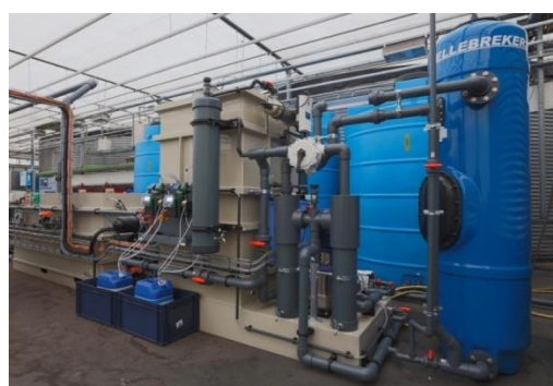
Figure 3-11. An example of a pilot installation for electrophysical precipitation in a horticultural greenhouse
