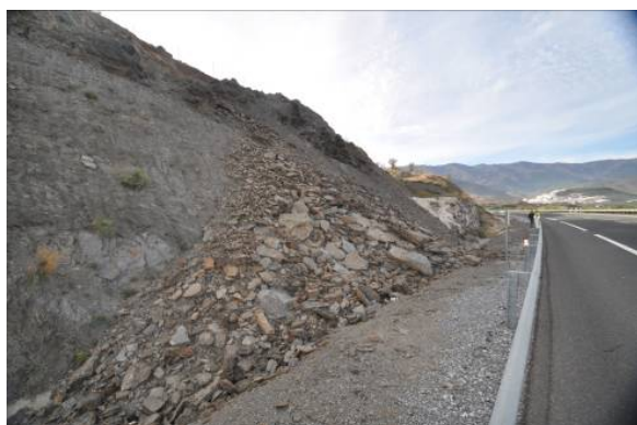
Fig. 6 Landslide in a road embankment in the kilometric point 339 belonging to the A92 dual carriageway, Spain.
